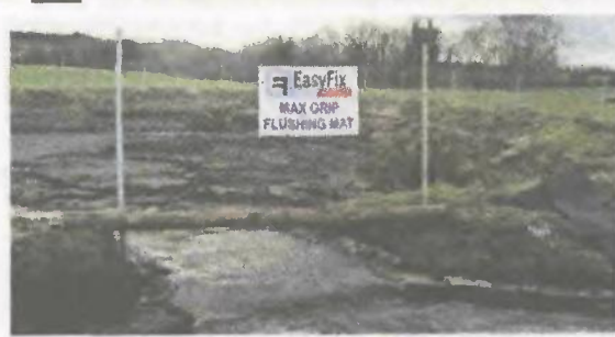
All waste water from the rubber is funnelled into a large earthen bank tank.
